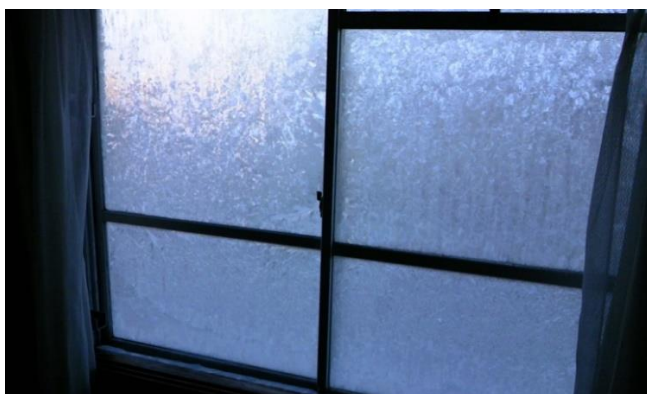
No heating – room windows frozen over midday
